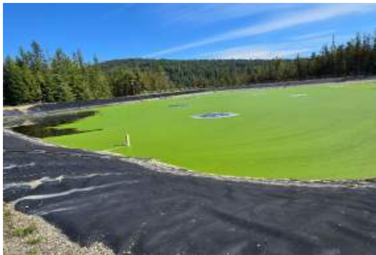
Effluent from our collection system (septic tanks) is pumped up to this aeration lagoon where sunlight and oxygen drive the biological decomposition of organic waste. DEQ looks for rips in the liner. We're good! This picture was taken in mid-September when the lagoon is down to its lowest level.
