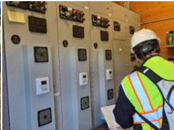
Inspecting our irrigation pump controls and activity records. The wastewater in the polishing lagoon is treated with chlorine and then sprayed in the surrounding forest.
